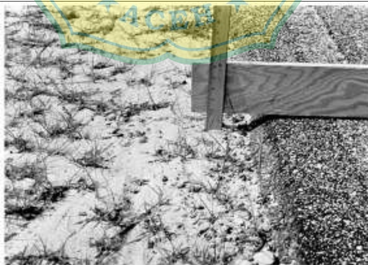
Gambar 2. 10 Penurunan bahu jalan ( lane/shoulder drop off ) Sumber : (ASTM D6433, 1995)
