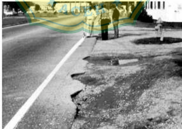
Gambar 2. 8 Retak Pinggir ( Edge Cracking ) Sumber : (ASTM D6433, 1995)
