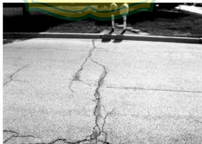
Gambar 2. 4 Retak blok ( block cracking ) Sumber : (ASTM D6433, 1995)
