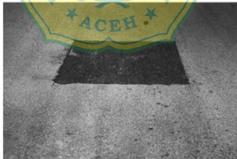
Gambar 2. 12 Tambalan dan galian utilitas ( patching and utility cut patching ) Sumber : (ASTM D6433, 1995)
