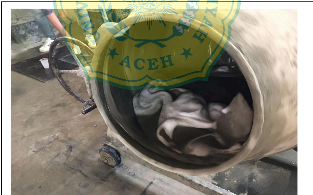
Gambar A.5.7 Pengecekan campuran beton busa didalam concrete mixer Sumber : Dokumentasi lapangan
