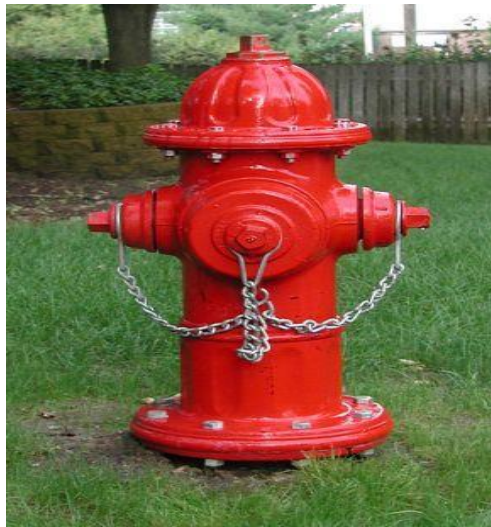
Gambar 4.21: fire hydrant Sumber: fire hydrant 2013
