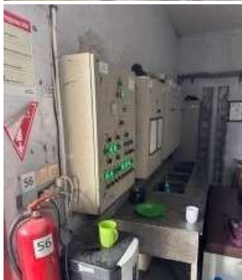
Panel Listrik & APAR
